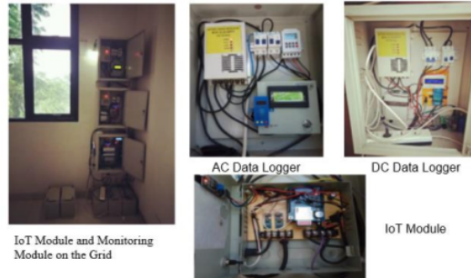
Fig. 5. IoT module and monitoring module on the grid
