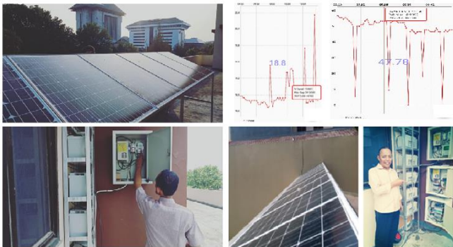
Fig. 4. Installation and monitoring of voltage and power on SHMG
