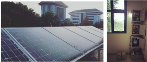
Fig. 1. Smart Home Micro Grid Installation
