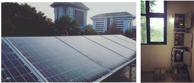
Fig. 1. Smart Home Micro Grid Installation
