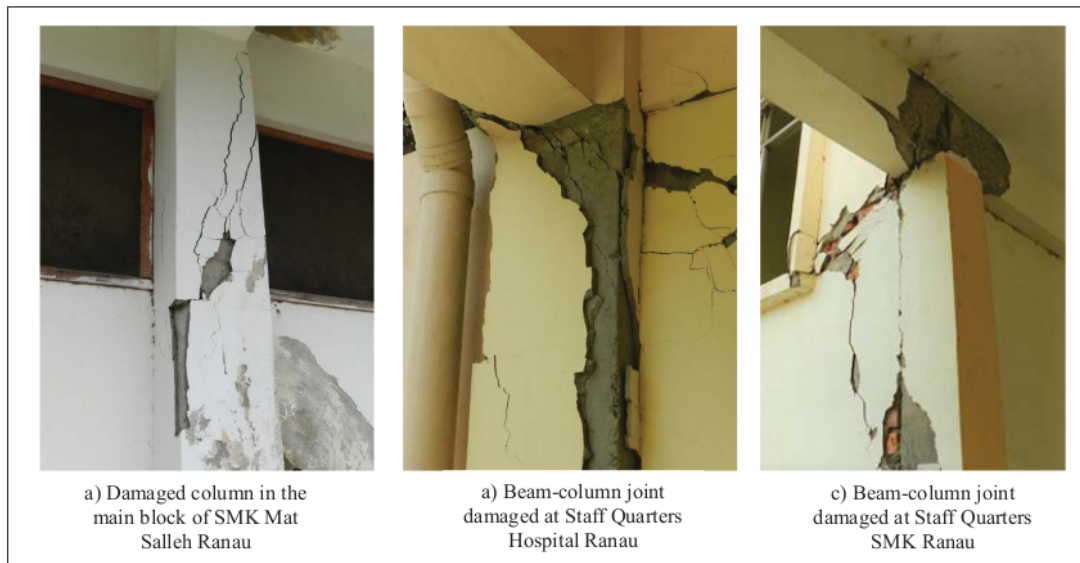
FIGURE 1. Structural damages at few school and public buildings after the 2015 Ranau Earthquake.
