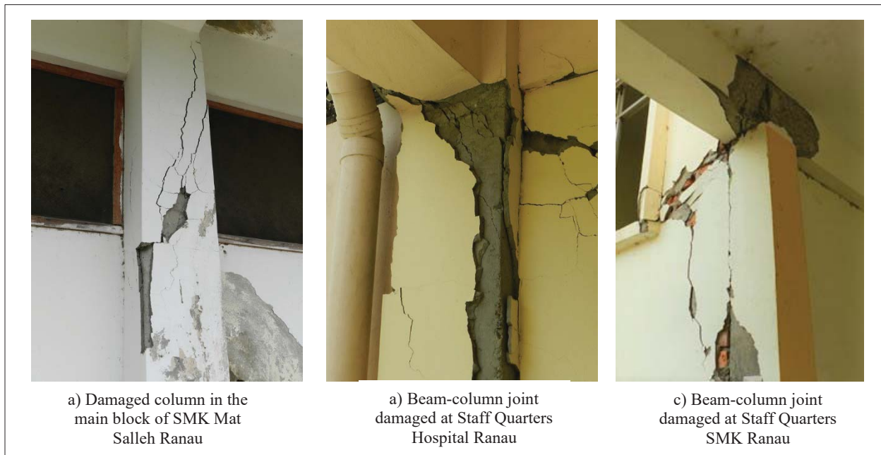
FIGURE 1. Structural damages at few school and public buildings after the 2015 Ranau Earthquake.
