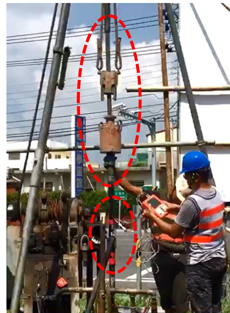
Figure 6. Auto-drop hammer system and hammer energy inspection arrangement adopted in the Phase I soil liquefaction study in Huwei & Tuku Township, Yunlin County, Taiwan.
