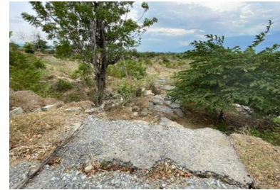
Photo 4'. After EQ (looking SW)
