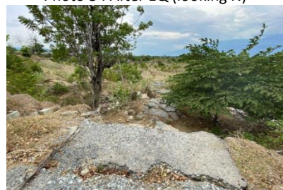
Photo 4'. After EQ (looking SW)
