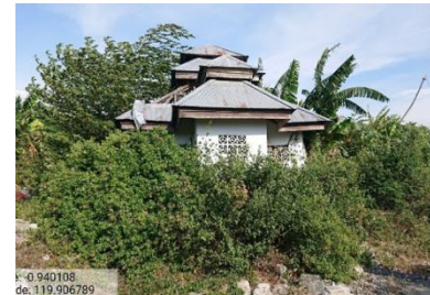
Photo 6'. After EQ (looking E)
