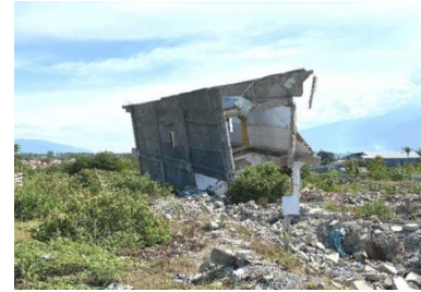
Photo 8'. After EQ (looking S)
