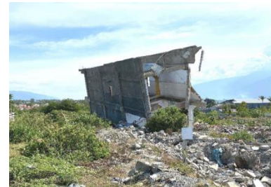
Photo 8'. After EQ (looking S)
