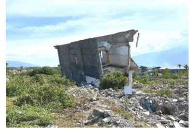
Photo 8'. After EQ (looking S)
