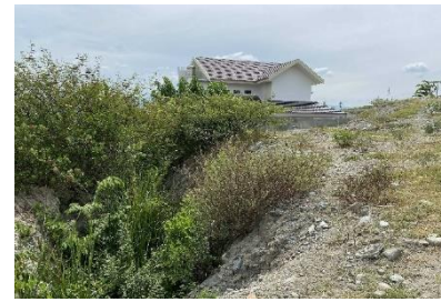
Photo 9'. After EQ (looking SE)
