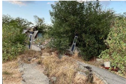
Photo 3'. After EQ (looking N)
