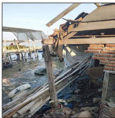
Figure 2. Residents' Houses Affected By Abrasion
