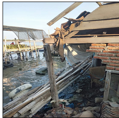
Figure 2. Residents' Houses Affected By Abrasion
