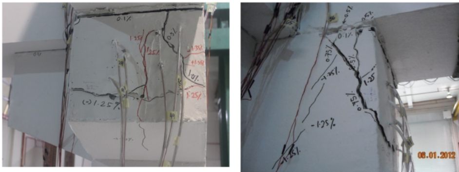
(a) Transverse cracks of 425 mm in length and cracks width of 10mm. (b) Diagonal cracks of 295 mm in length and an 8 mm opening of the gap occurred at the corbel
