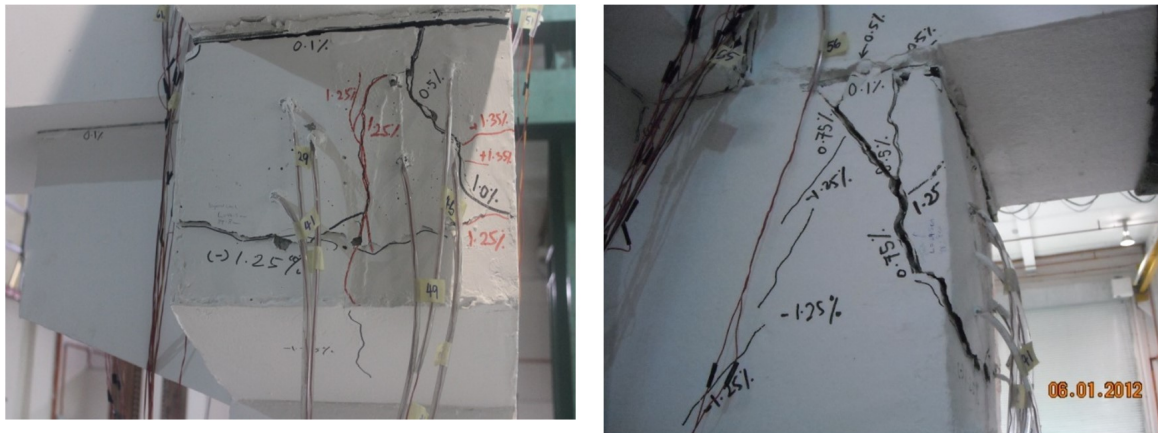
(a) Transverse cracks of 425 mm in length and cracks width of 10mm. (b) Diagonal cracks of 295 mm in length and an 8 mm opening of the gap occurred at the corbel
