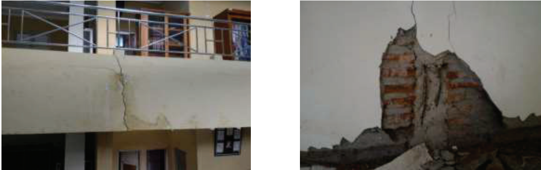
FIGURE 1. Some failure of beam and wall in Home Economics Department, Universitas Negeri Semarang
