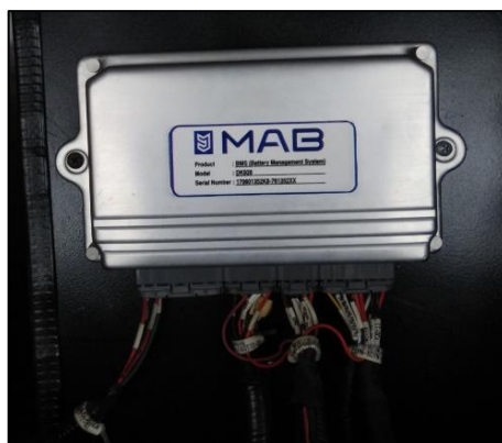
Gambar 2.3 Battery Management System
