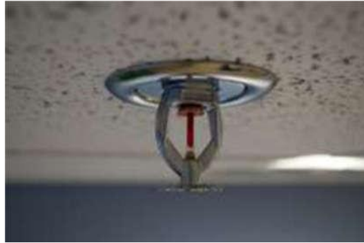
Gambar 4.30 Sprinkler Sumber : allegiantfire.com
