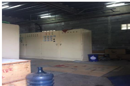
Gambar 2.69 Ruang Genset Marina Convention Center Semarang
