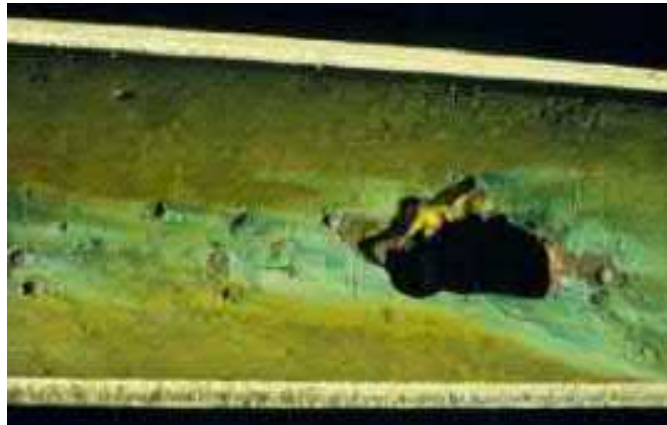
Gambar 2.5 Korosi Erosi (Utomo, 2009)
