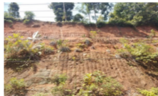
Figure 5. Landslide Prone Areas in Way Krui Sub-district Source: Photo of Meri, March. 2019
