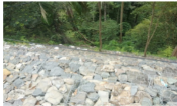
Figure 4. Landslide Mitigation Efforts at Way Krui
