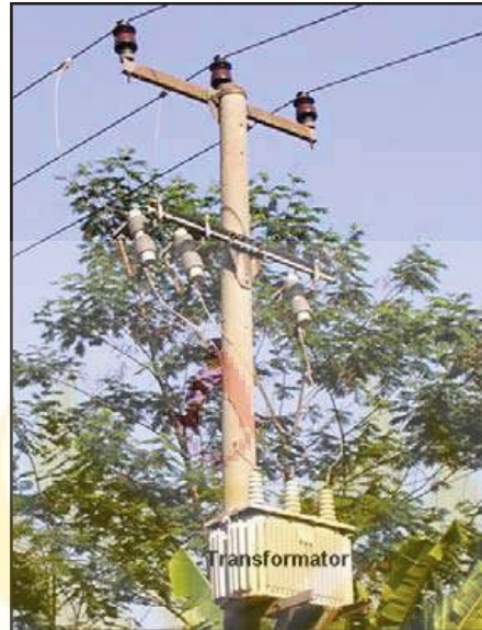
Gambar 2.3 Transformator Distribusi Tipe Tiang
