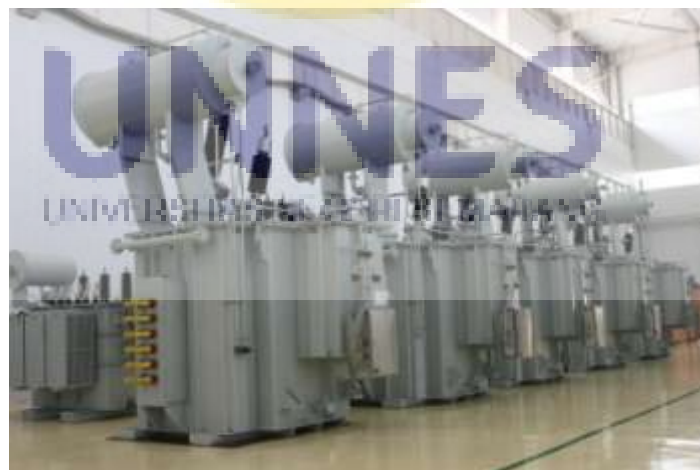
Gambar 8 Pendingin Transformator Type ONAF
