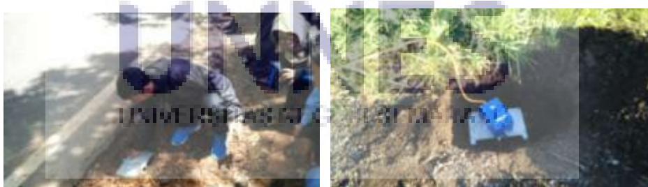
Gambar Perletakan Alat Sensor Seismic Monitoring
