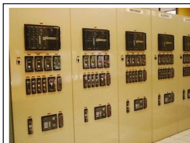
Gambar 2.8. Panel Kontrol Rele.
